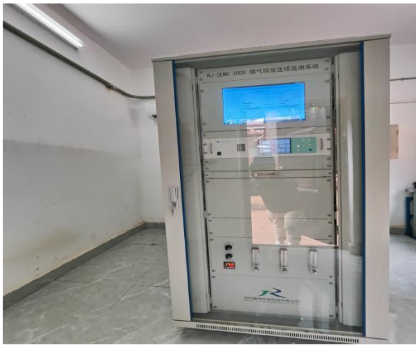
250m 2 烧结机机头烟气脱硫出口在线监测设施
