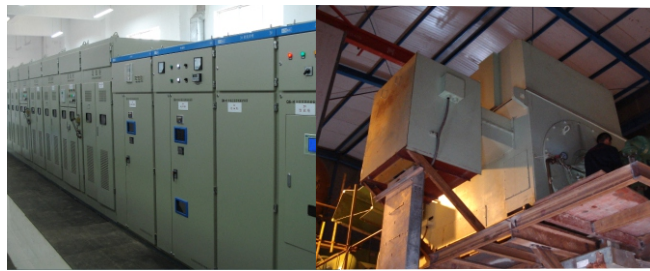
紫金铜业20万吨铜冶炼制氧压缩机系统 软起动装置型号: ATA QB-H10/18000 电机: 上海电机厂 负载: 制氧压缩机 (CAMERON) Zijin Copper 200,000 tons of copper smelting oxygen compressor system Soft Starter Model: ATA QB-H10/18000 Motor: Shanghai Electrical Machinery Co.,Ltd. Load: Oxygen Compressors (CAMERON)
