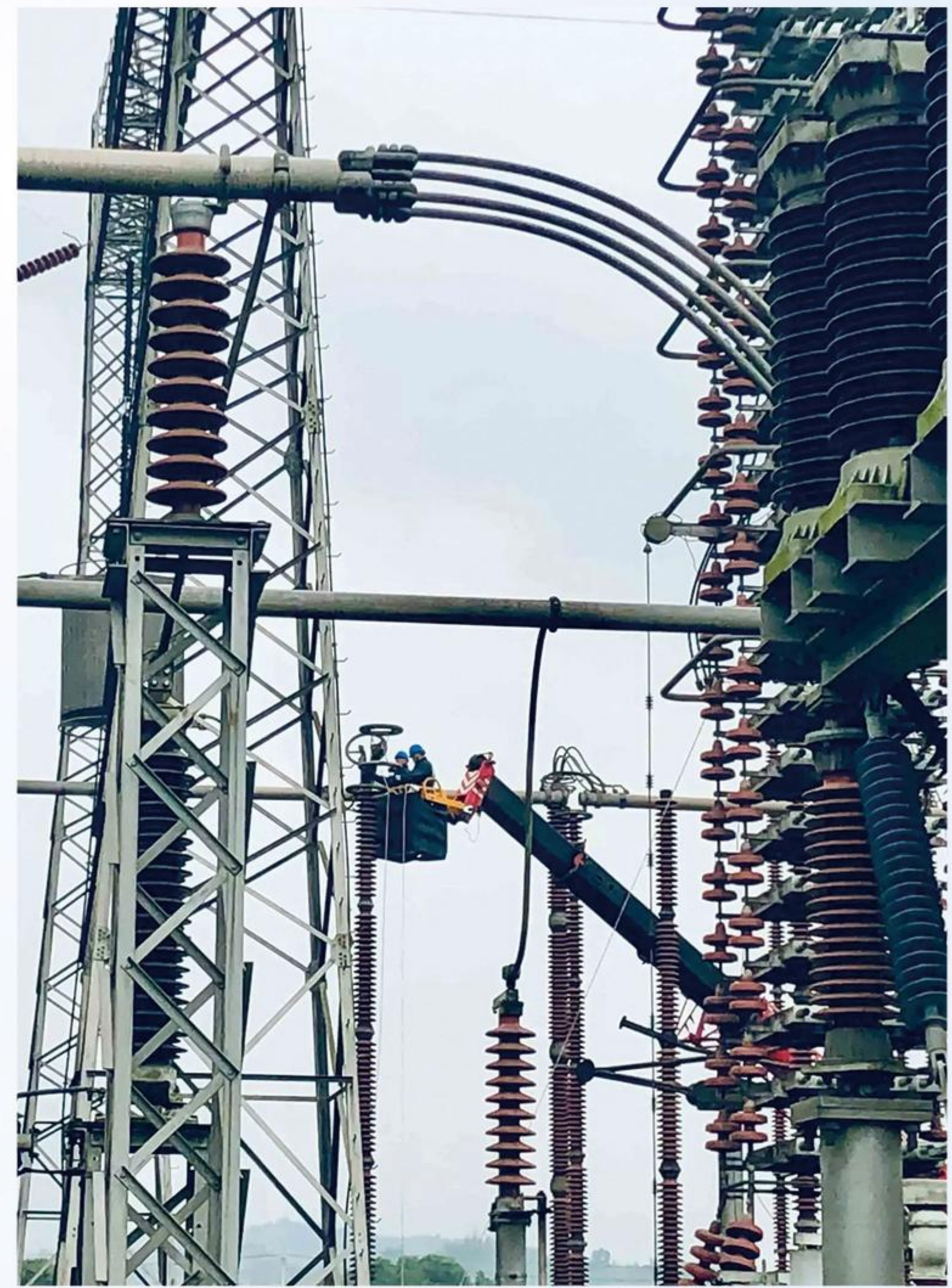
输变电 Power Transmission
